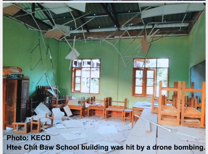
Htee Chit Baw School building was hit by a drone bombing.
